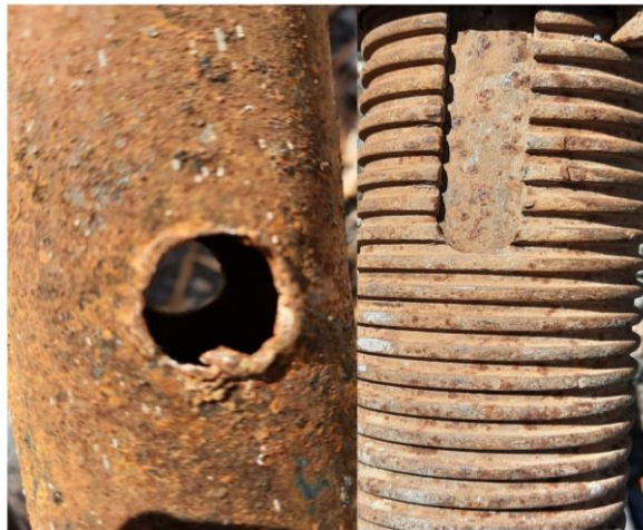
Figure 1: Representative images of engineering equipment damage due to corrosion.
