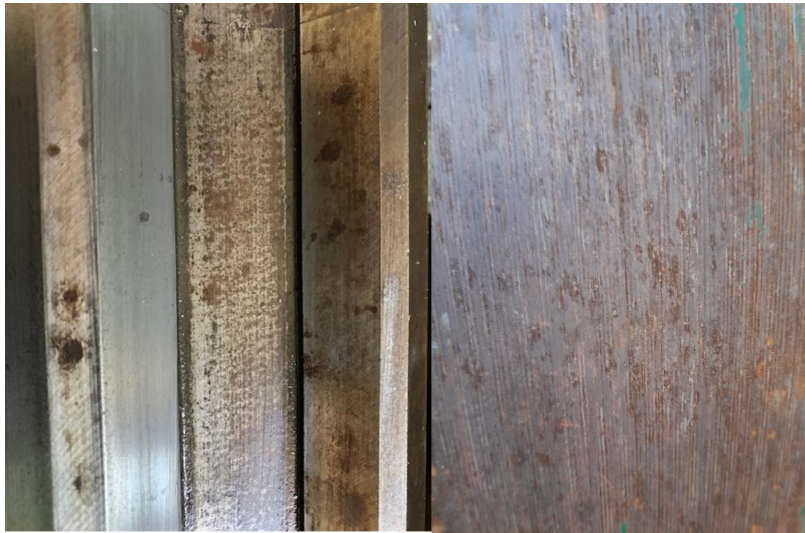
Figure 3: Representative images showing the combined effect of corrosion and sliding in engineering parts.
